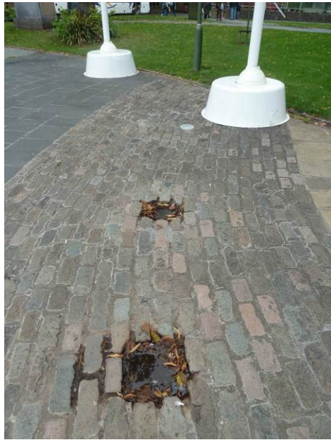
Repairs needed to cobbles in Priory Square
