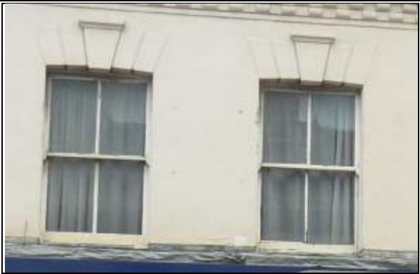
Later Sash Windows to Number 96
